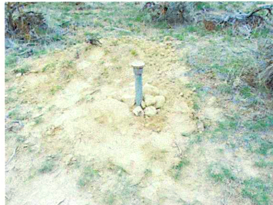
Buried monument to within 8 inches of the surface. Original stone was placed upside down with the tip above the surface on the West side of the Brass Cap. Using the only stone available in the general area I placed a very small mound around the monument.
